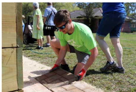
STPN Folsom Office Manager Joe Schonacher lays a paving stone on the perimeter of the new Safe Haven community garden. (Photo by Tim San Fillippo / STHS)
