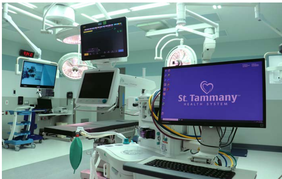
A look at one of the 12 state-of-the-art surgery suites at the new St. Tammany Health System Surgery Center, which also boasts 24 private pre-op rooms, 18 recovery rooms and 15 rooms with overnight-stay capabilities. (Photo by Tim San Fillippo / STHS)
